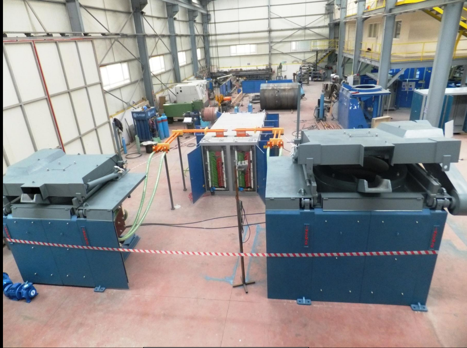
Duet Power System Furnace View
