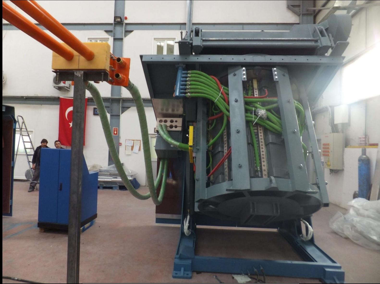
Furnace Energy Connection And Push Out System View
