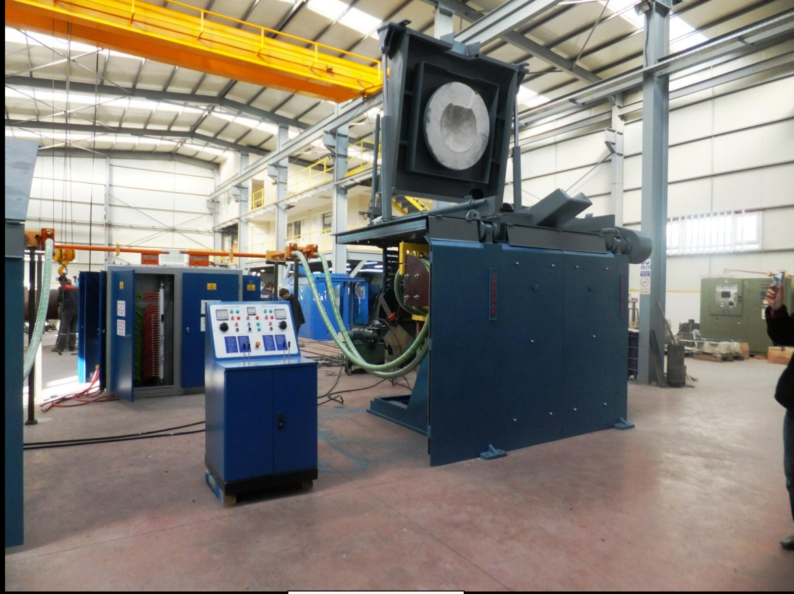
Furnace Cover View
