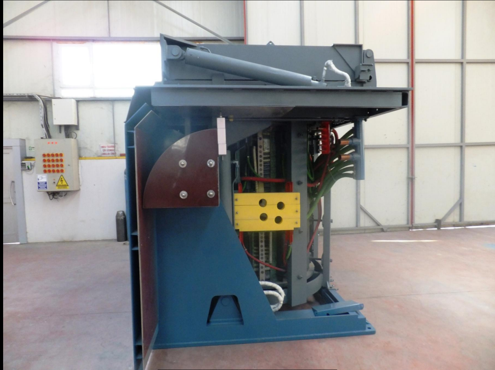
Furnace Energy Connection View
